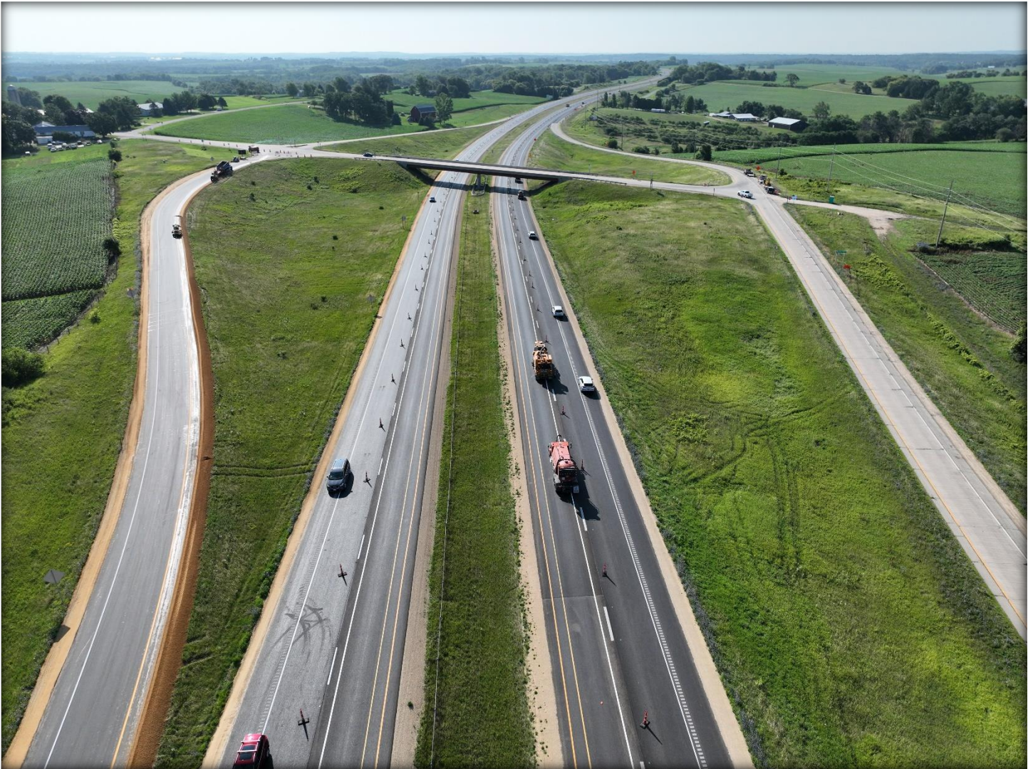
Photo above: Crews continue finishing items just west of CTH PD. All lanes of US 18/151 from CTH G to Mount Horeb are scheduled to reopen on Wednesday, July 26
