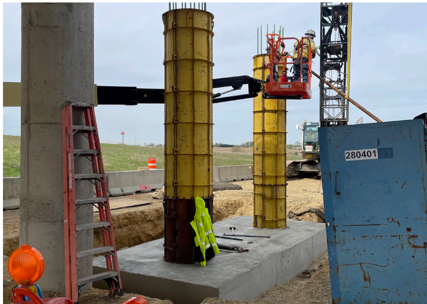
Above: Pier column construction at County G/ Dairy Ridge Road over US 18/151
