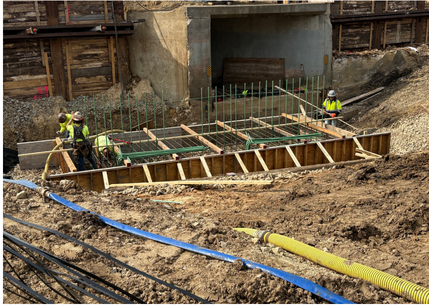
Above: Wing wall footing construction at the Military Ridge Trail box culvert north of US 18/151
